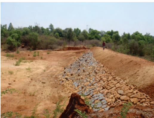
Nala bund with upstream stone pitching for storing runoff, ground water recharge and supplemental irrigation in Tumkur district
