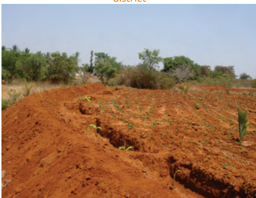
Trench-cum-bund in red soil for in-situ moisture conservation with Banana plantation in trenches in Tumkur district
