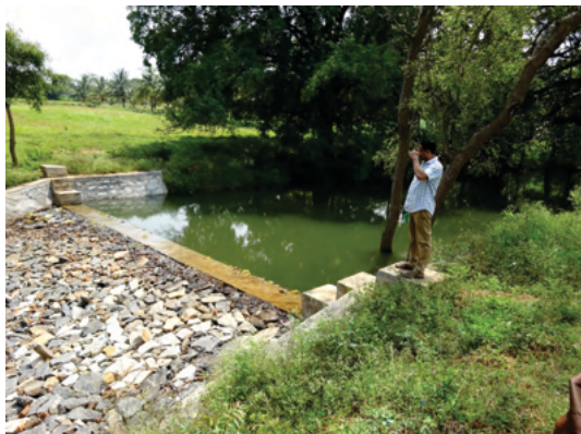
Masonry check dam across nala with water ponding upstream side constructed for storing runoff and erosion control in Chamrajnagar district
