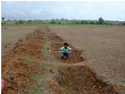
Trench-cum-Bund in hard rock soil for in-situ moisture conservation and erosion control in Bidar district
