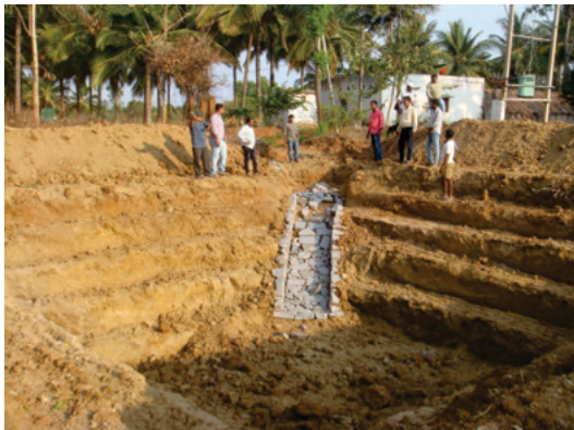
Dugout farm pond constructed to harvest rainwater for life saving irrigations in Tumkur district
