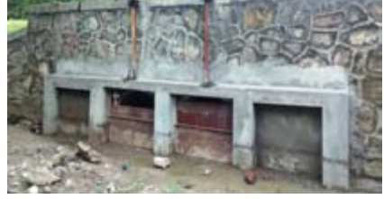
(f) Pipe culvert with gates (Kolahpuri style)
