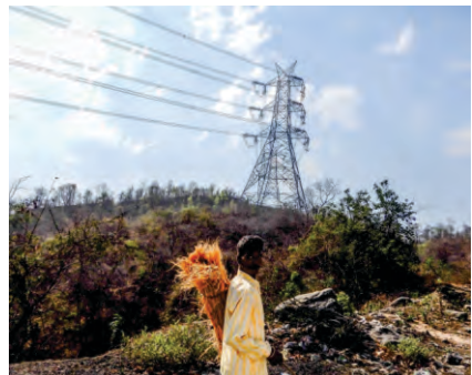
The transmission line – passing through forest
